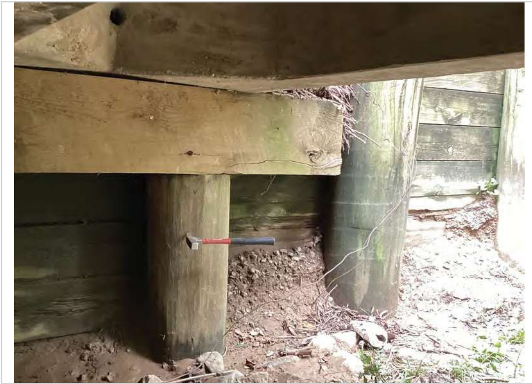
Abutment 2 cap above pile G 1/16" grain crack
