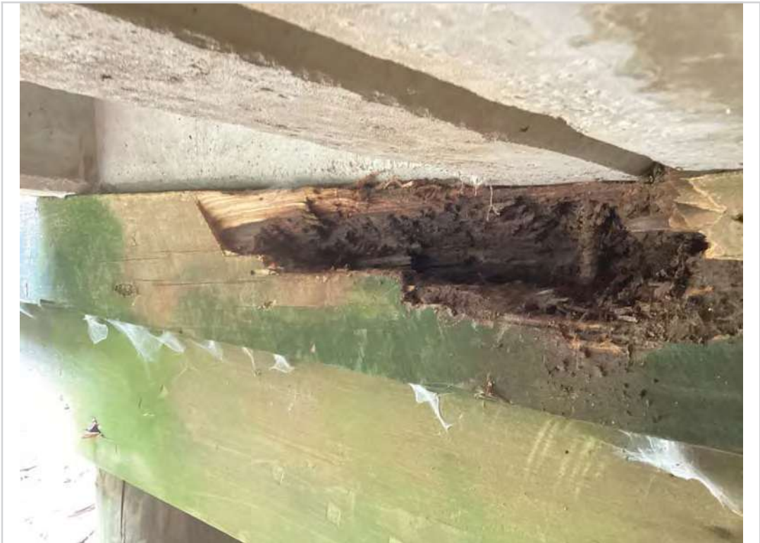
Bent 1 front side decay
