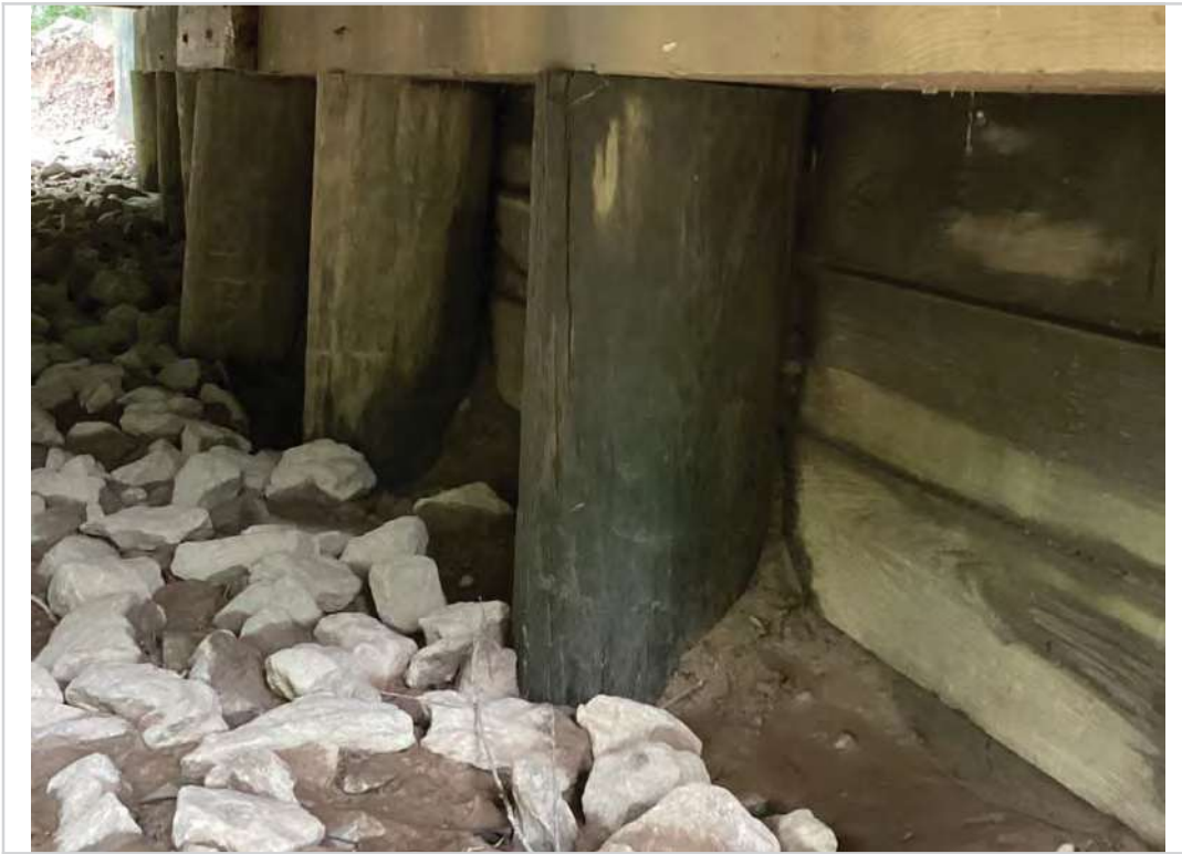
Abutment 2 pile F grain cracks
