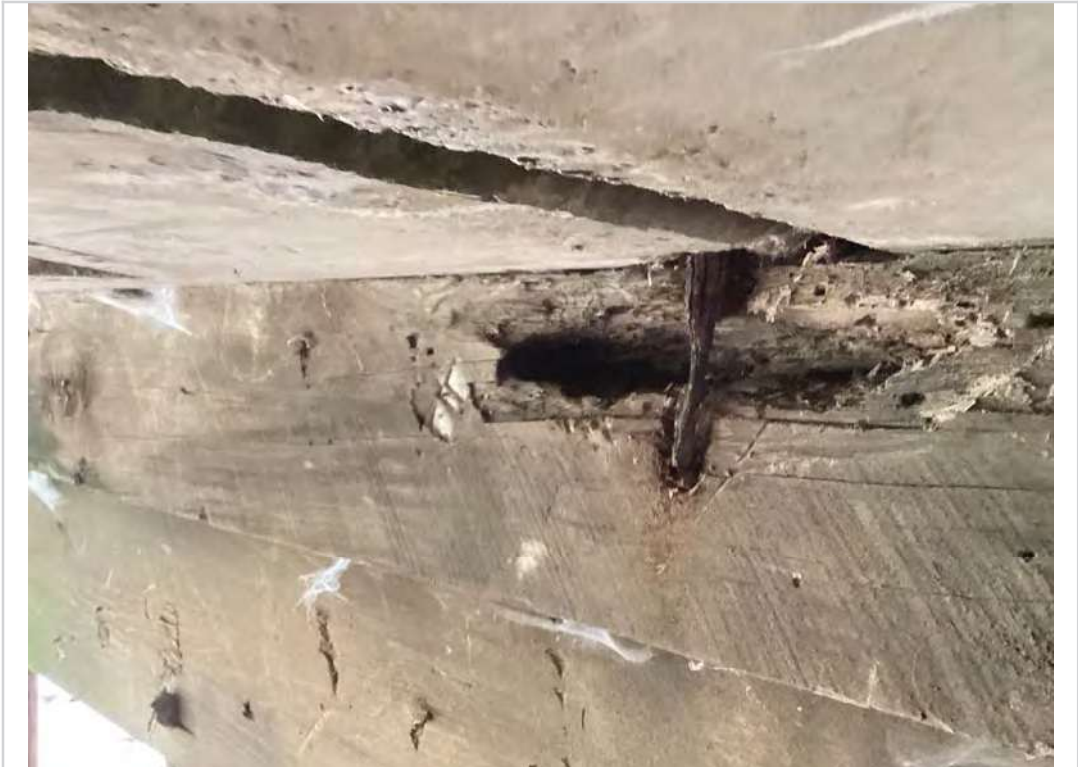
Bent 1 front side decay
