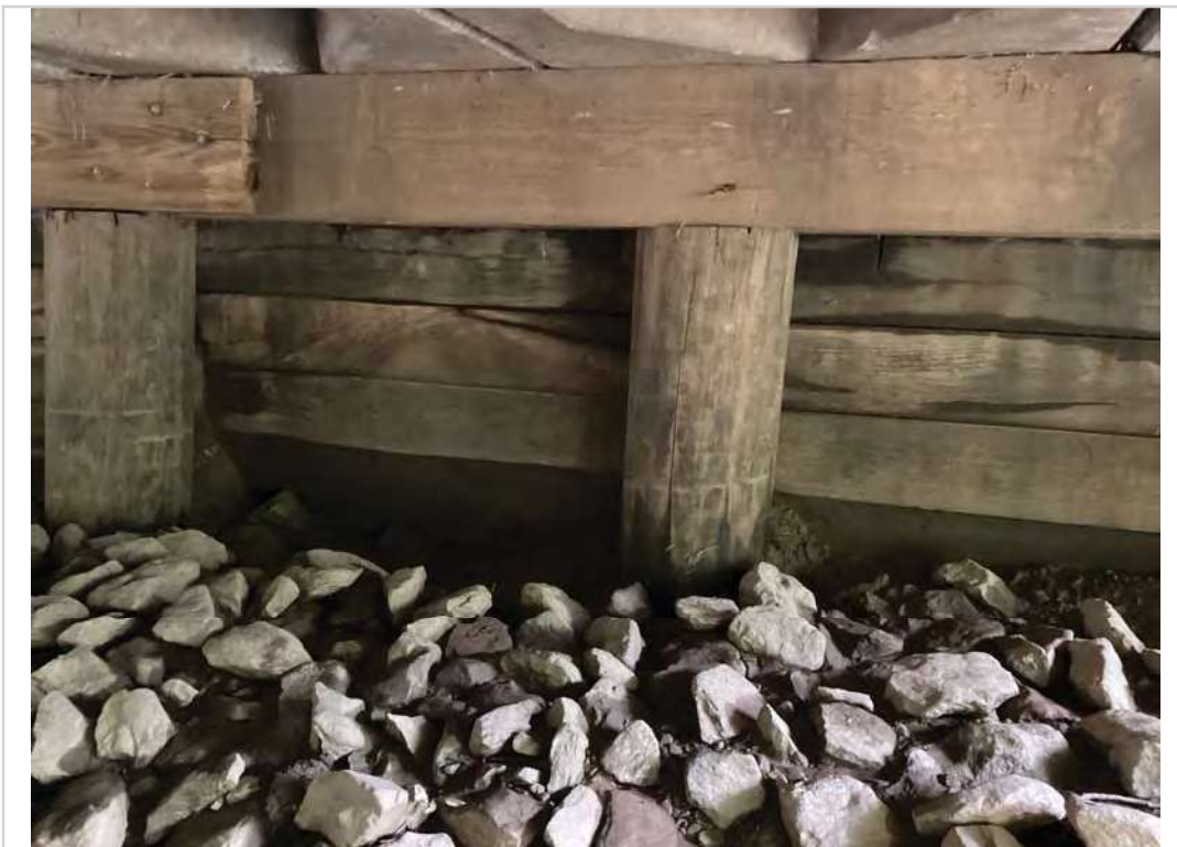
Abutment 2 breast wall between piles D and E beginning to break/ splinter
