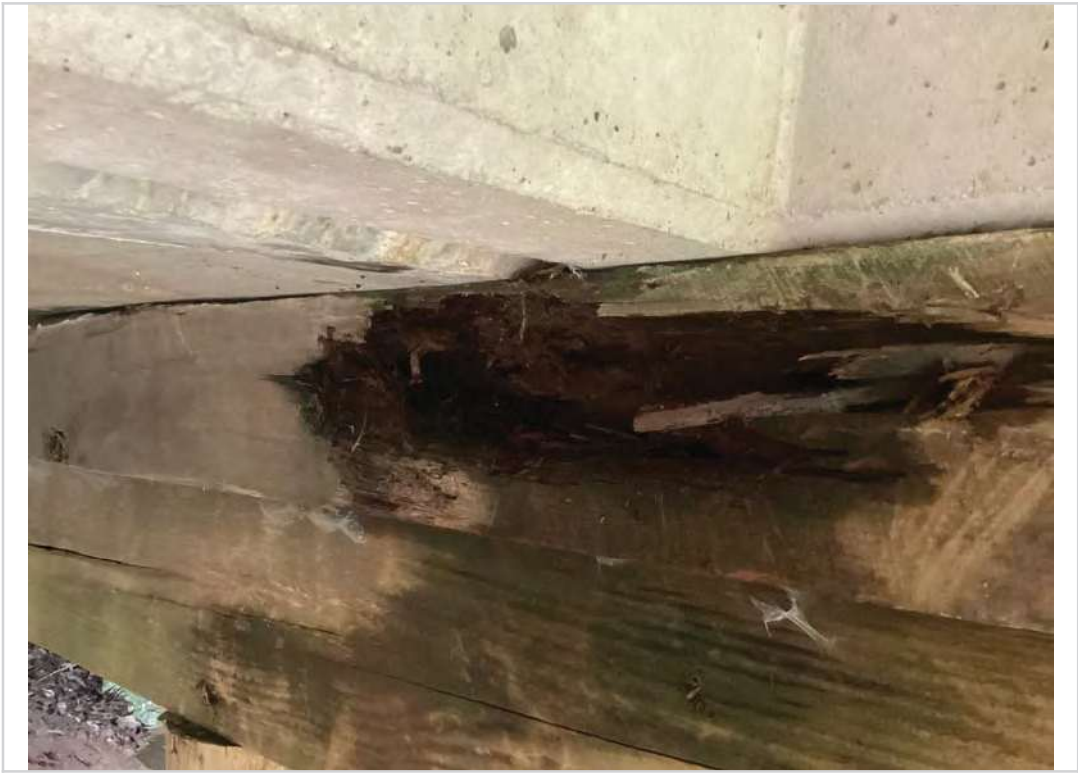
Bent 1 front side decay
