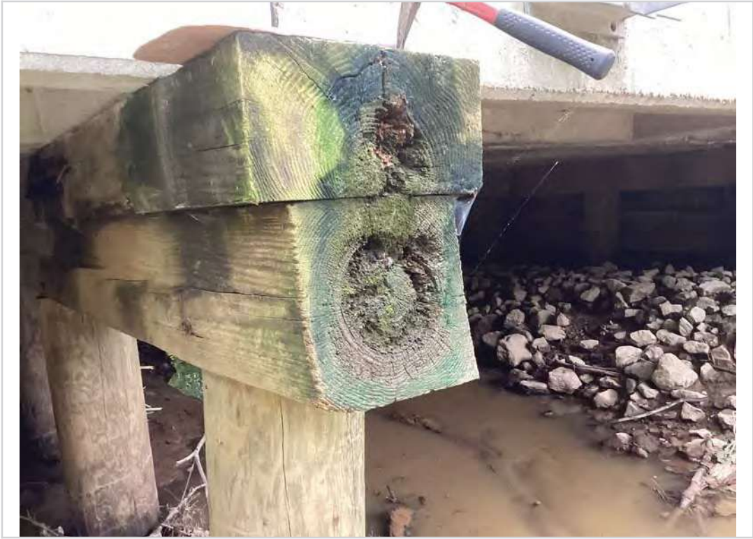
Bent 1 right side decay
