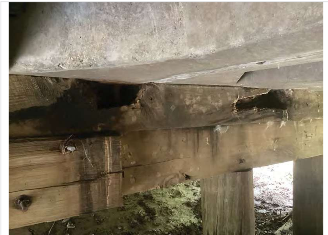
Bent 1 decayed areas rear side
