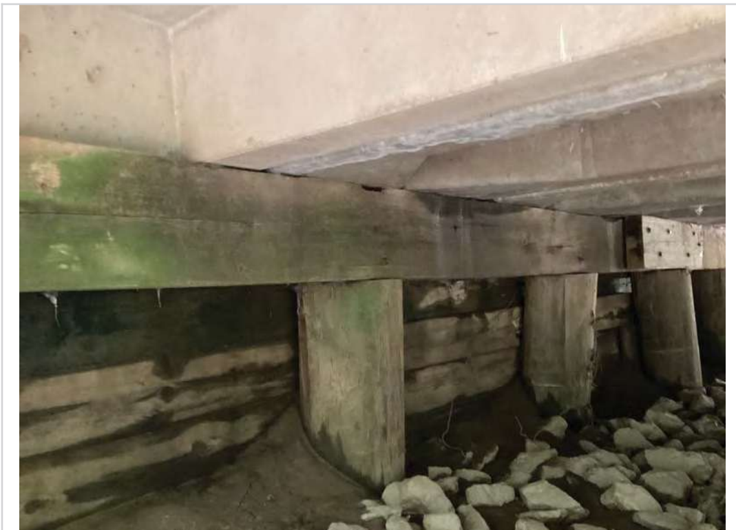
Abutment 2 cap splintered area
