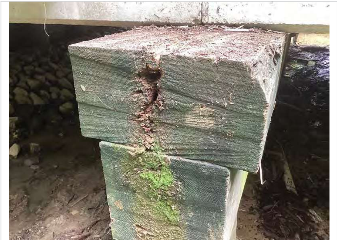
Bent 1 left side decay
